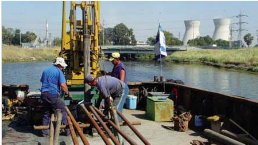
Pumping in the Kishon River. Photo: Gil Gutman, Kishon River Authority.
